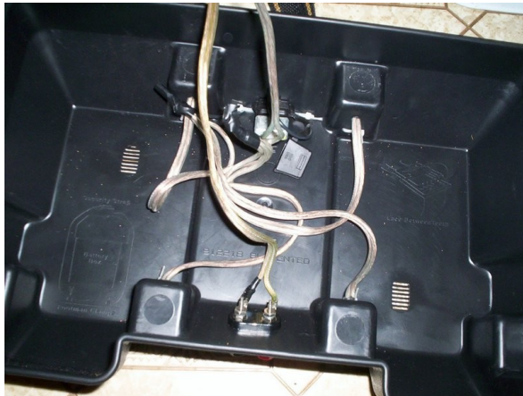
Inside view with fuse holder in upper middle
